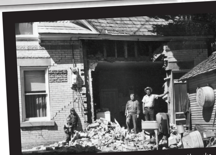
Damage from the 1962 M 5.7 Cache Valley earthquake (Ariel Benson, University of Utah Library)
